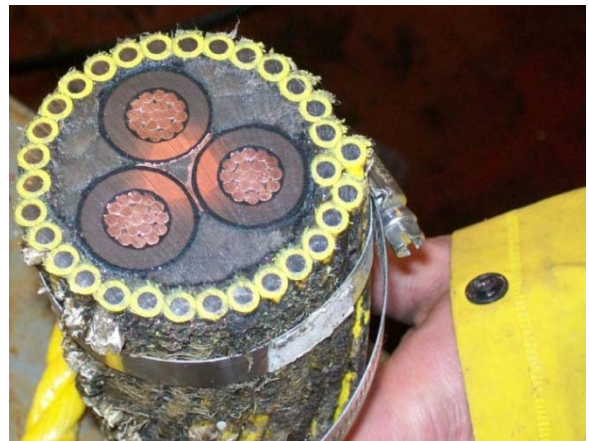
Marine cable (discolored insulation and copper tape shield deterioration visible)
