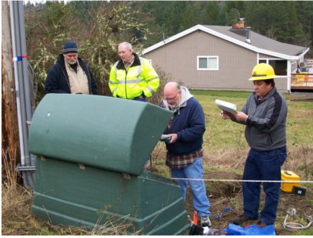
Fault locating from Anderson Island side
